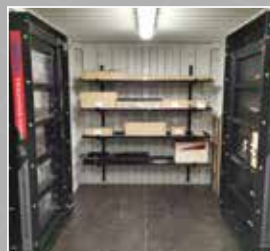
Storage for spare parts
